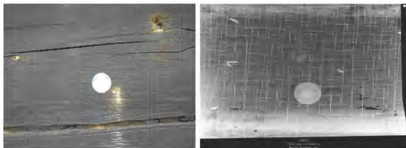
Fig. 12: Attacked wooden element sample combined with plaster and metal mesh; the larva occurrence is marked with a red oval. Measured on 1 June 2012, Mlýn, Kozlovice, Czech Republic.
